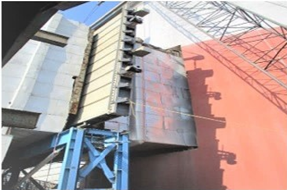
Duct Damper Alignment
